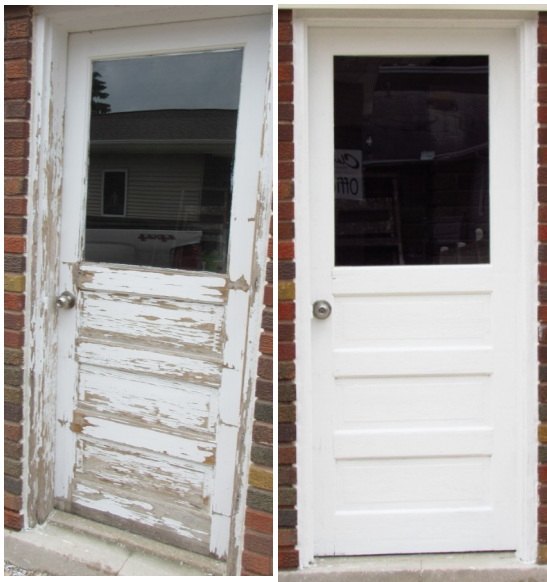
A door several years past needing a fresh coat of paint.
